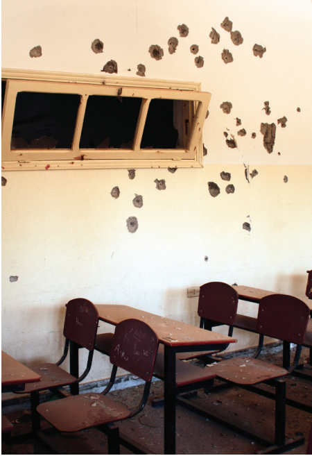
Bullet holes in a classroom at El Jeel Eljaded School, Libya
