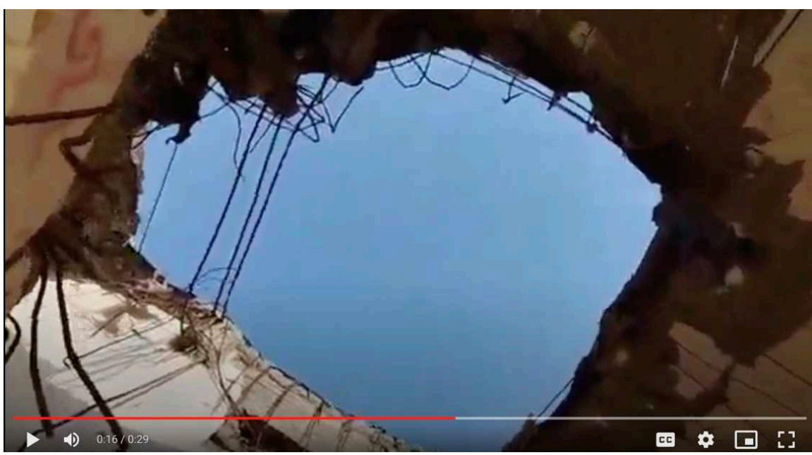
image 28: an installed shot from a video clip shows a hole caused by aerial bombardment of the roof of the school building.
