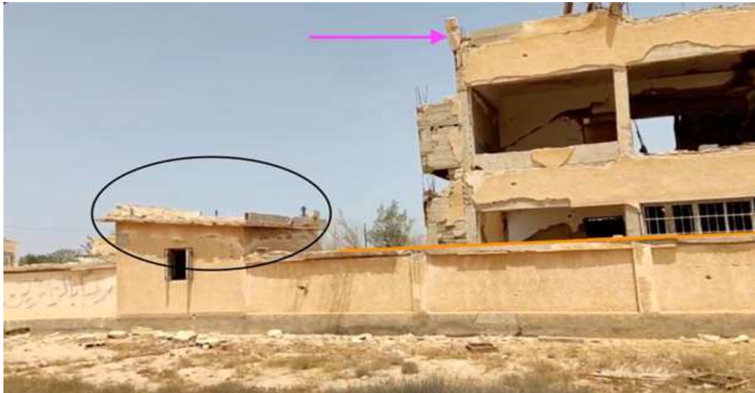
Image 4: Image of the actual dilapidated building, the south wall and a small building on the edge of the school.
