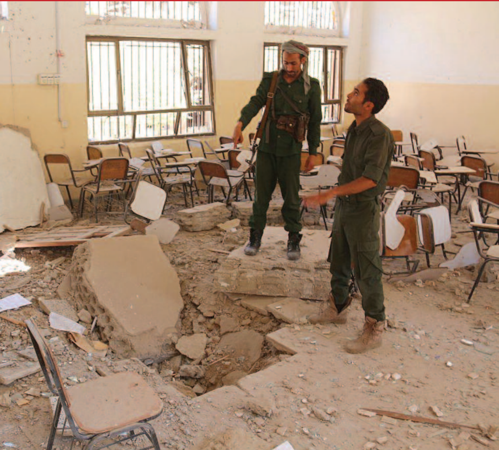
Houthi fighters inspect a school building damaged by Saudi-led coalition airstrikes in Ibb's Varim, Yemen on April 23, 2015.
